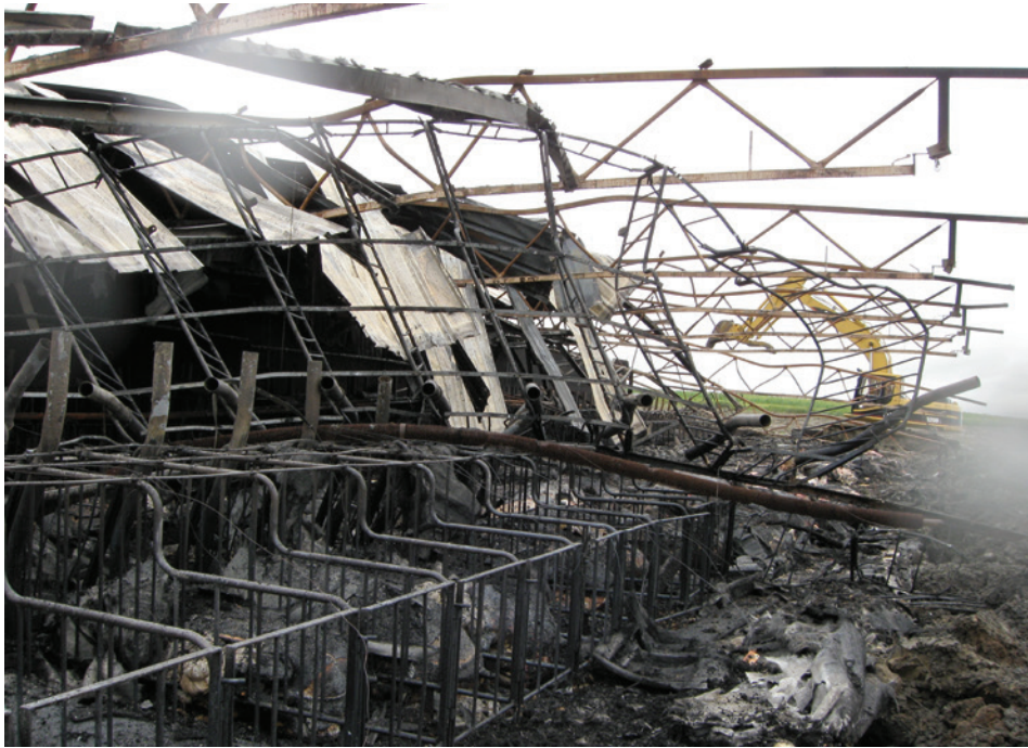
The aftermath of a massive pig barn fire. Sows were unable to escape from their gestation crates and perished in the fire.
